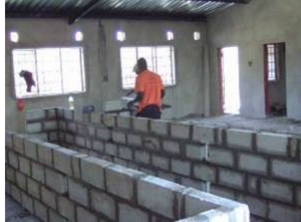
Laboratory Project in progress at Makeni Ecumenical Centre. The concrete tables under construction.
