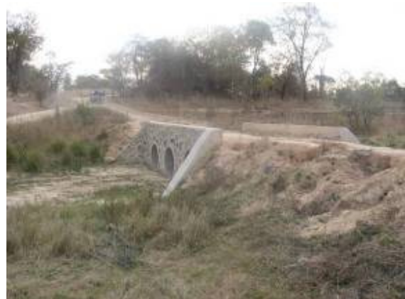
The bridge (constructed in 2013) damaged during the early rains of 2014
