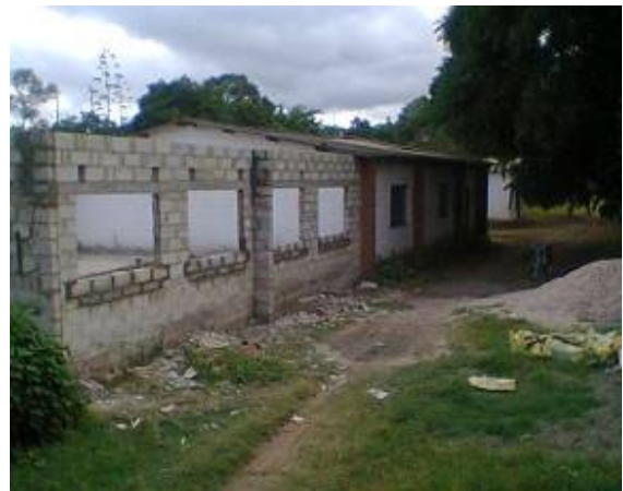
The School Laboratory under construction with the help of the Friends of Makeni in the Netherlands
