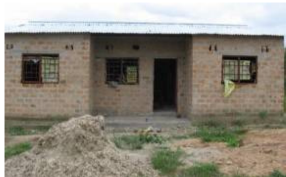
The second teacher's house, built with support from the Friends of Makeni and the Chisamba Member of Parliament in Mwomboshi
